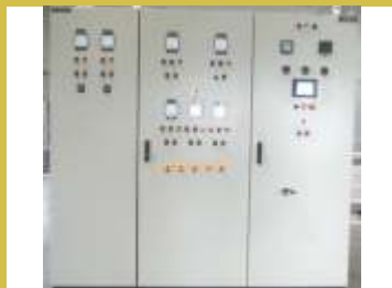
VFD/ PLC Panels
